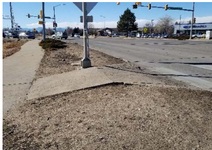
Curb ramp with PROWAG compliance issues at Ken Pratt Boulevard and Sunset Street intersection.
