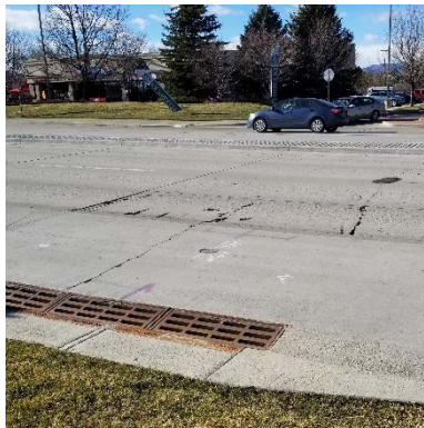
Spalling of concrete pavement along Hover Street.
