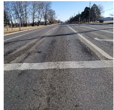
Rutting of asphalt pavement along Nelson Road at the intersection of Hover Street.
