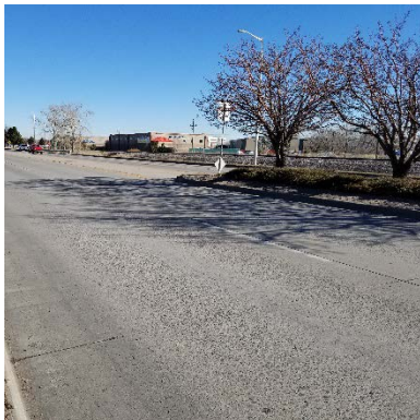
Surface wear of concrete pavement along Ken Pratt Boulevard.
